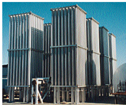
FIGURE 1—Ambient air vaporizer back-up system.
