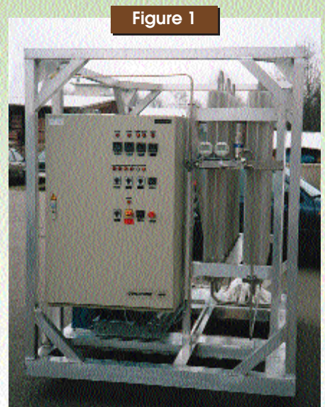
The electrical control cabinet of the pump/vaporizer skid.
