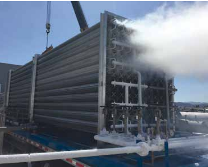
Figure 5 – Horizontal fan ambient in operation
