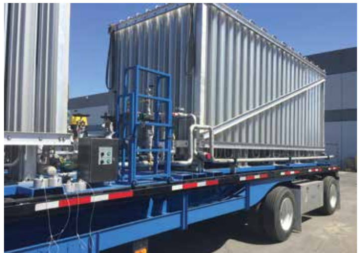
Figure 2 - Controls, ladder and hose racks
